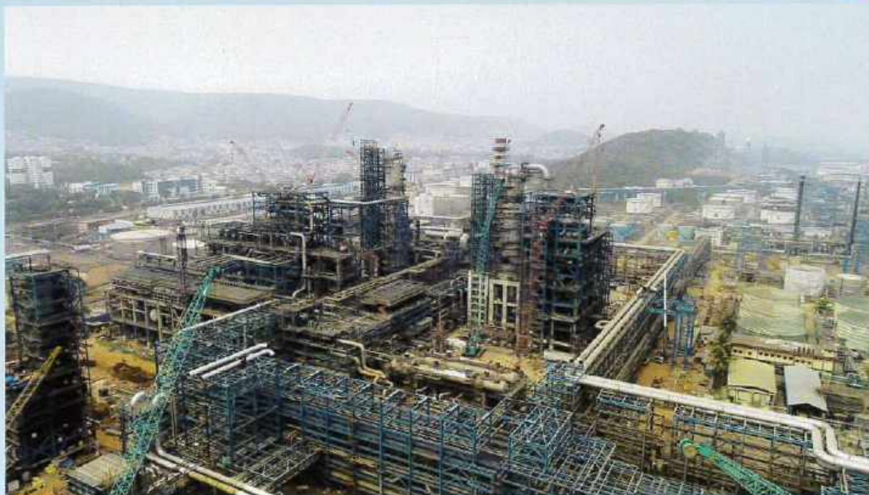
CDU Overall View of Visakh Refinery Modernization Project
